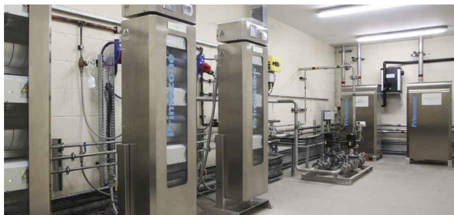
Primozone ozone installation at Acomb Landing - 3 GM18 ozone generators, 2 DM ozone destructors and a dissolution module.
