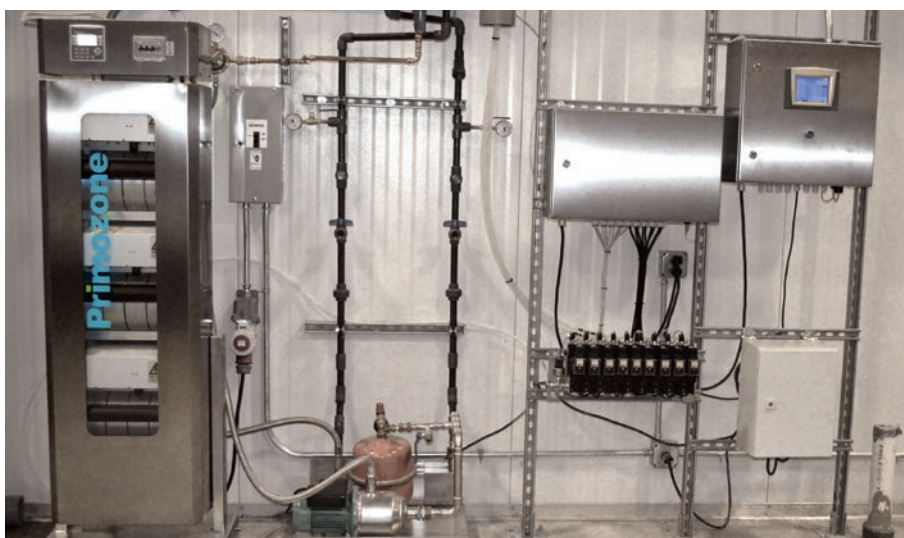
Complete installation at Bell Aquaculture with a Primozone® GM18 ozone generator, Primozone® ODM ozone distribution module, Primozone® system controller and a heat exchanger.
